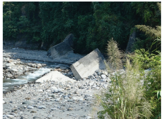
Figure 1:Groynes constructed (and subsequently destroyed by high river flows) in an unsuccessful attempt to train the river away from the BFAL factory site
