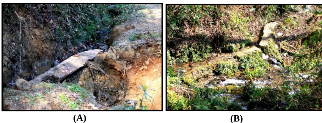
Photo 2: (A) Overflow & leakage of irrigation channel. (B) Damaged irrigation channel
