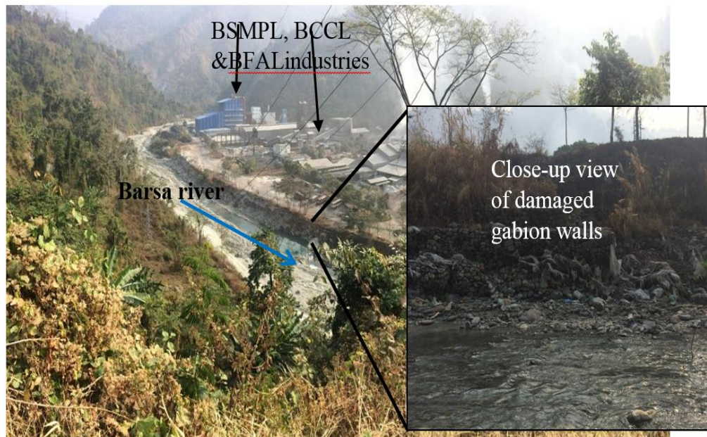
Figure 31. Photo shows damaged gabion walls along the left bank of Barsa river below the industries.
