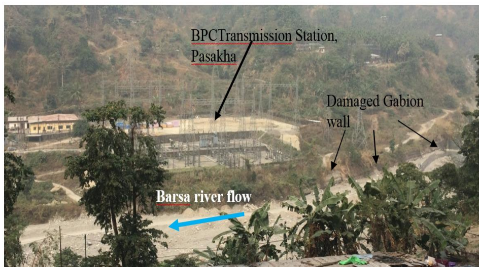
Figure 30. Pasakha transmission station with disturbed gabion wall along the right bank of the river.
