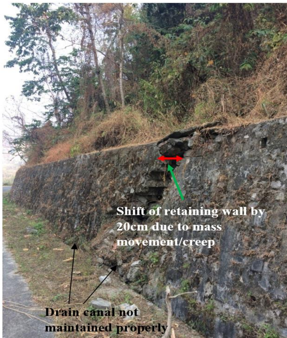
Figure 17. Displacement of retaining wall due to a mass movement.
